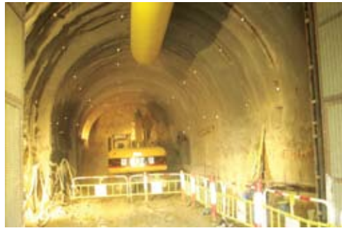
Top left: Tunnel excavation for West Island Line Underground Magazine at Victoria Road.
