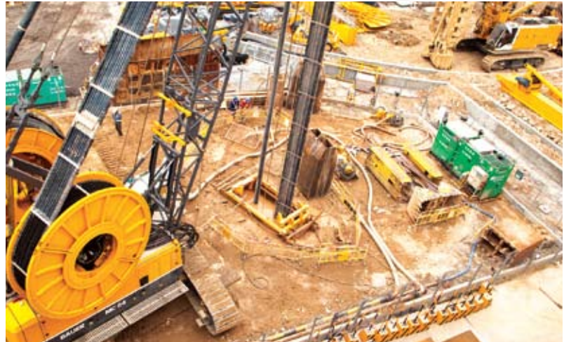
Top right and bottom: HATS stage 2A comprises the construction of three deep tunnels totalling 12km in length and eight shafts.
